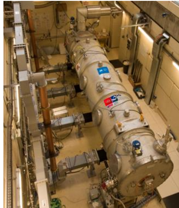
ESS cryomodule installed in the test stand at Saclay
