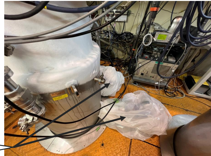
They were installed beside the VT cryostat
