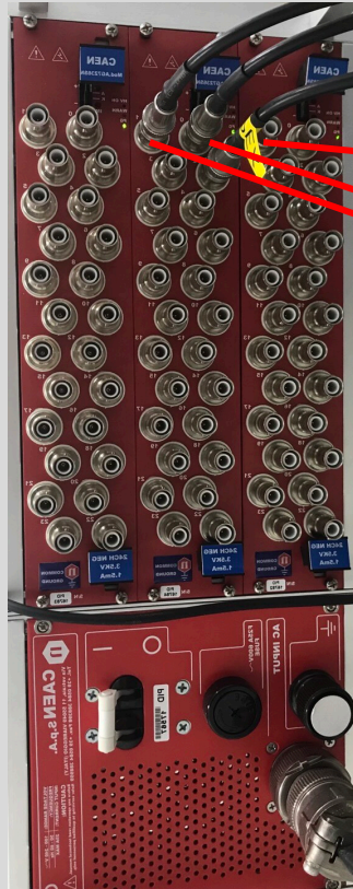
▲ Rear view of HV supply
